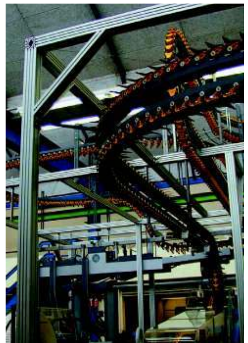
Newspaper handling system
