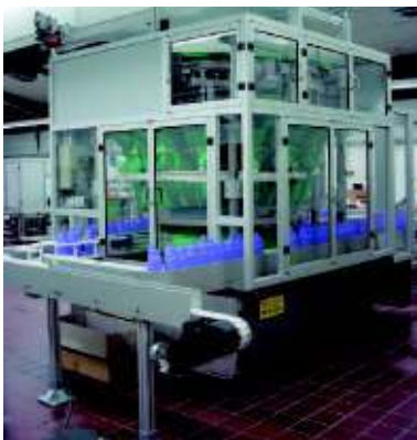
Clean room housing
