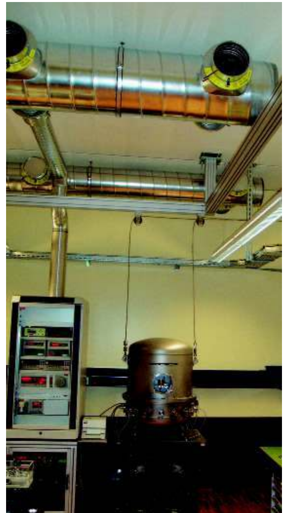
Laboratory equipment with ceiling grid system
